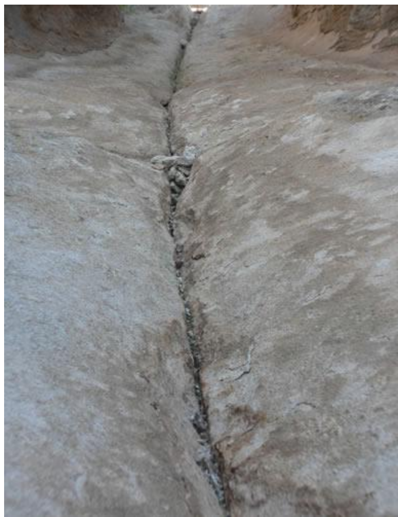
Figure 7 – Fracture in the middle of one of the "streets" at City of Rocks State Park.
